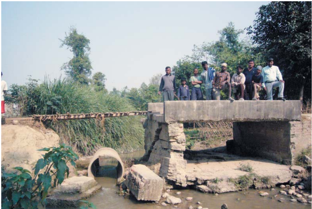
Local community standing on a bridge destroyed by flood, Singyali VDC, Mohottari District, Nepal
