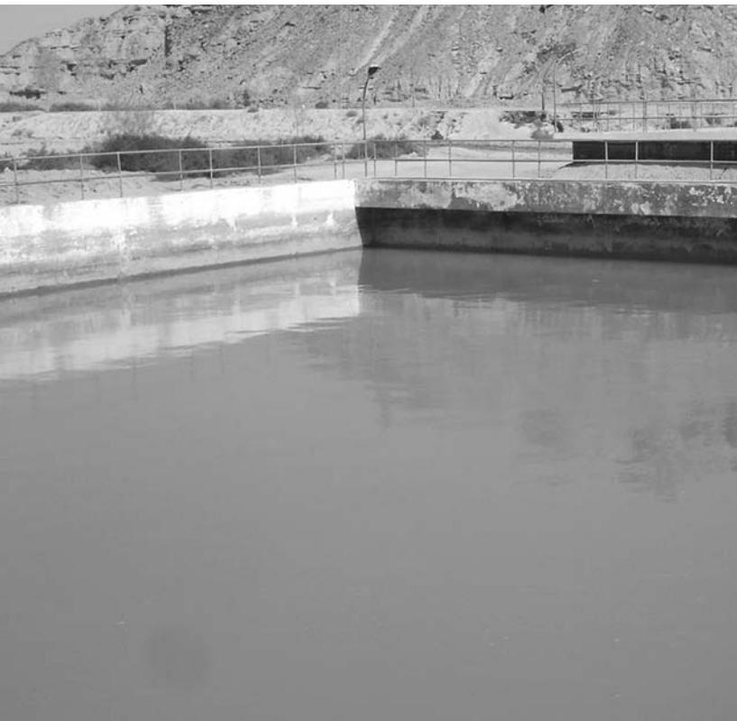
Sand filter bed for supplying drinking water from Ankra Kaur Dam reservoir to Gwadar Town and surrounding areas
