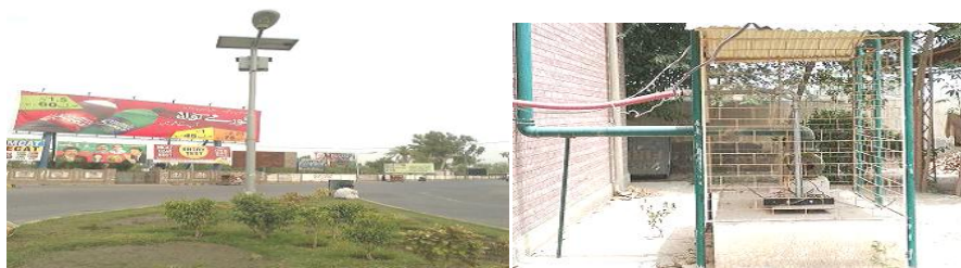
Solar lights and water pump installed in Muzaffargarh
