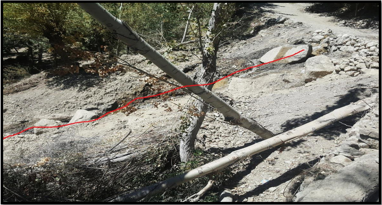
Figure 7: Visible Cracks observed during Field Visit
