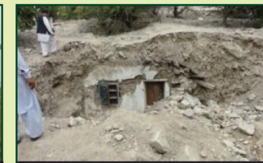
Fully damaged house at Garam Chashma
