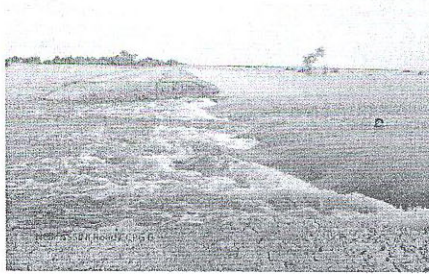
BREACH IN APPROACH ROAD
