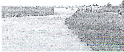
FLOOD WATER ENTERING IN TO KC AFTER BREACHING
